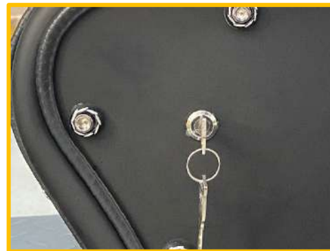
Figure 2 – Speed override switch (OFF)
